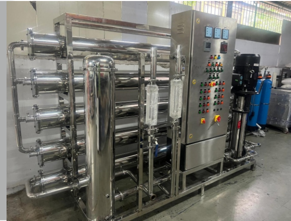
R O Plant
